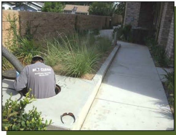
Vacuuming out of media filters.
