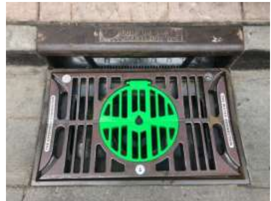
Image 5 - Installed DIF-C with diverter screen and optional OGB grate (access hatch closed)
