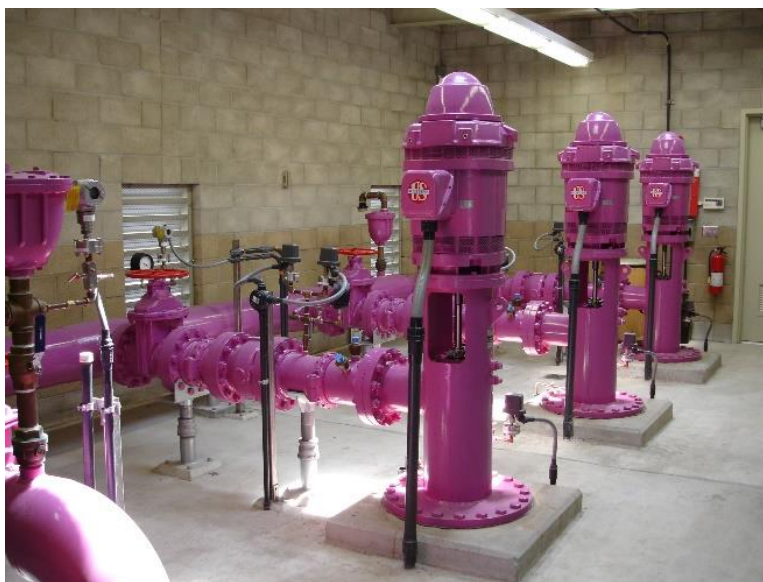
Calavera Hills Pump Station (60 HP)
