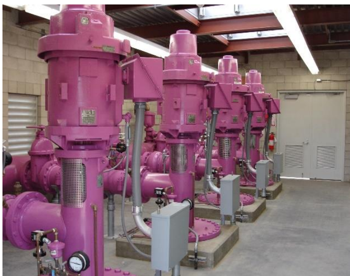
The 150 HP Twin "D" Pump Station, which helps deliver recycled water to CMWD customers.
