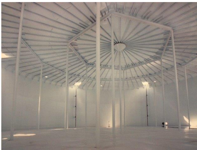
CMWD's 8.5 MG D3 Reservoir
