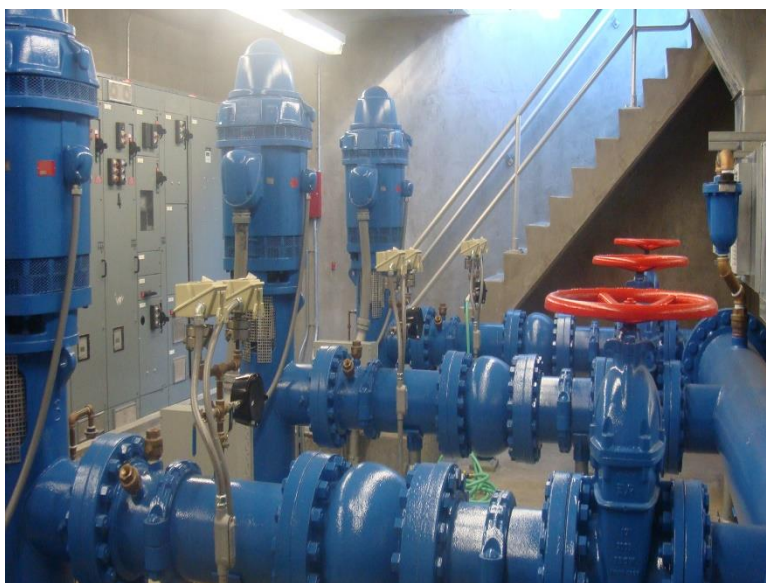
The 125 HP Bressi Potable Water Pump Station
