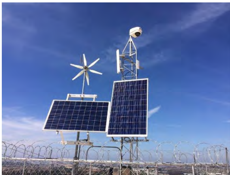
Solar and wind power used at CMWD's off-grid Santa Fe II facility
