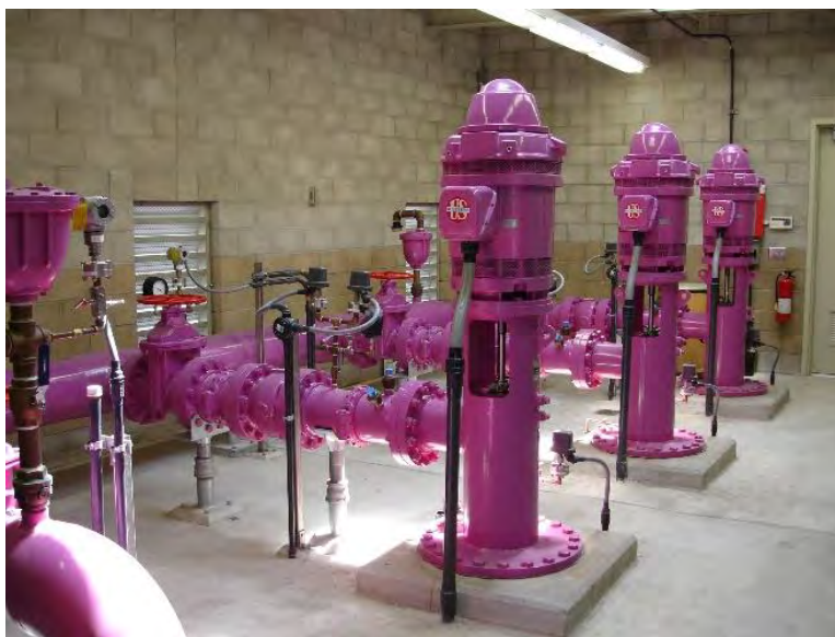
Calavera Hills Pump Station (60 HP)
