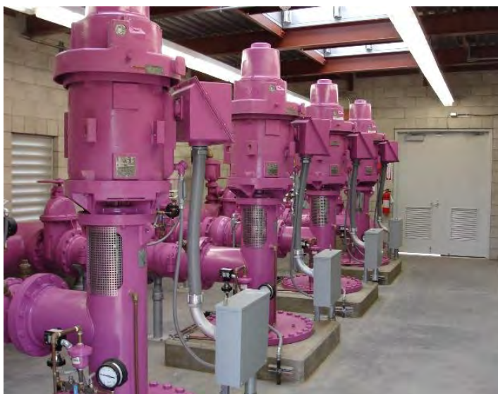
The 150 HP Twin "D" Pump Station, which helps deliver recycled water to CMWD customers.
