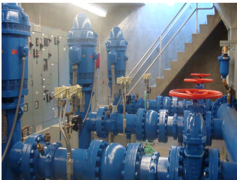
The 125 HP Bressi Potable Water Pump Station
