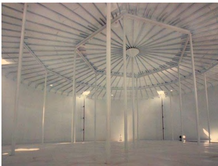
CMWD's 8.5 MG D3 Reservoir
