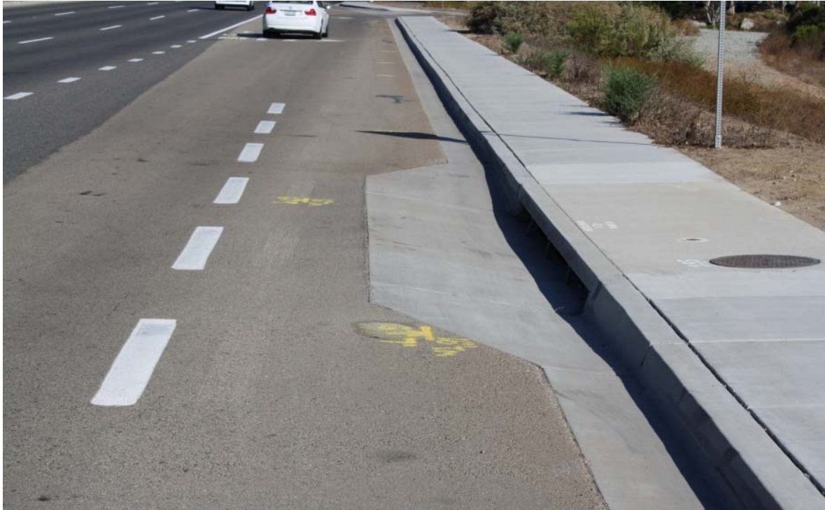
The Public Utilities Department reduced the grade of storm drain depressions to increase comfort for cyclists.
