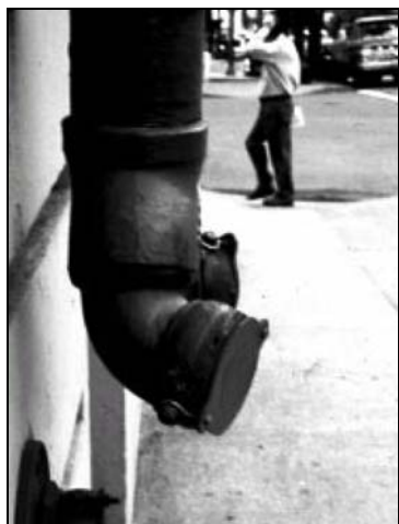
Elements such as standpipe systems may project into the Frontage Zone. Care must be taken to assure compliance with the ADA.
