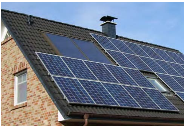
The City of Carlsbad is looking to solar technology to reduce energy demand from city facilities, and eventually, from households and businesses, too.
