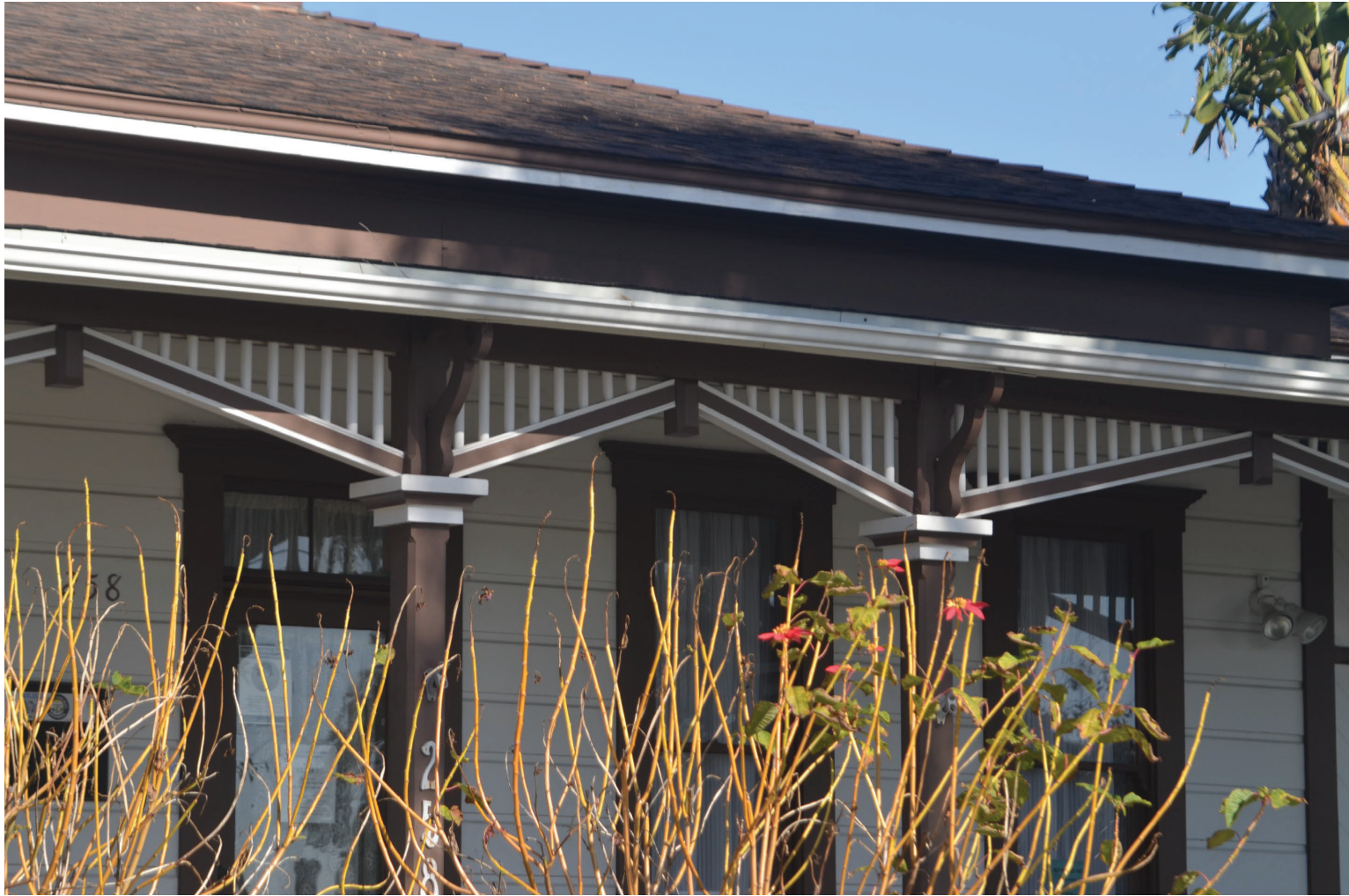
Note the siding , fascia boards and architectural trim-work ,especially the spindle porch ornament
