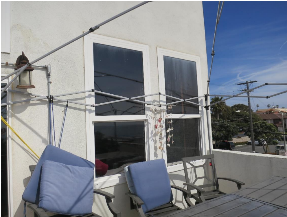
Figure 25. Detail of windows on south façade of 2689 Garfield St., view to southeast
