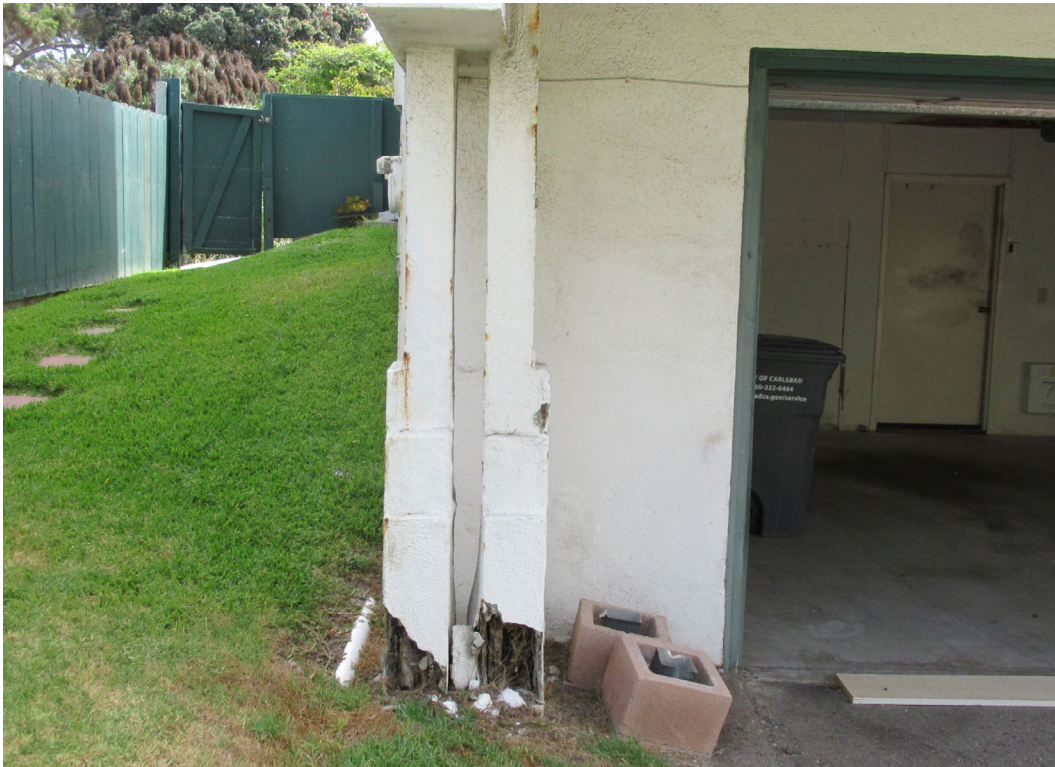
Photo 5: One of four pairs of damaged structural columns on the west façade.
