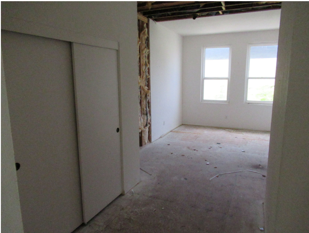
Photo 16: Bedroom 2C showing missing finishes.
