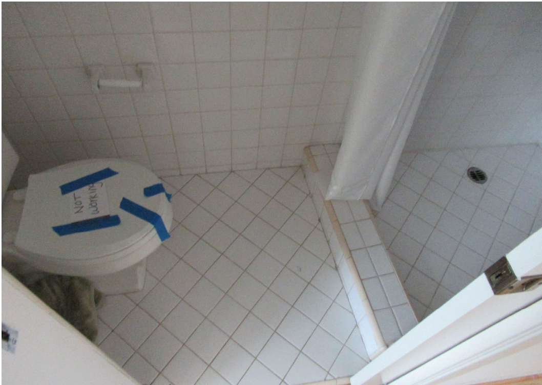
Photo 30: Original ceramic tile wall and floor finishes in the toilet/shower room of Bathroom 1B.
