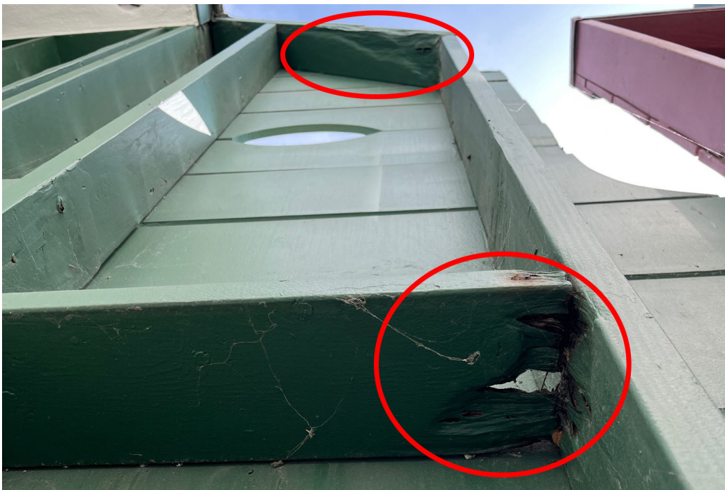
Photo 10: Additional wood damage (circled) in the structural framing of the false front.
