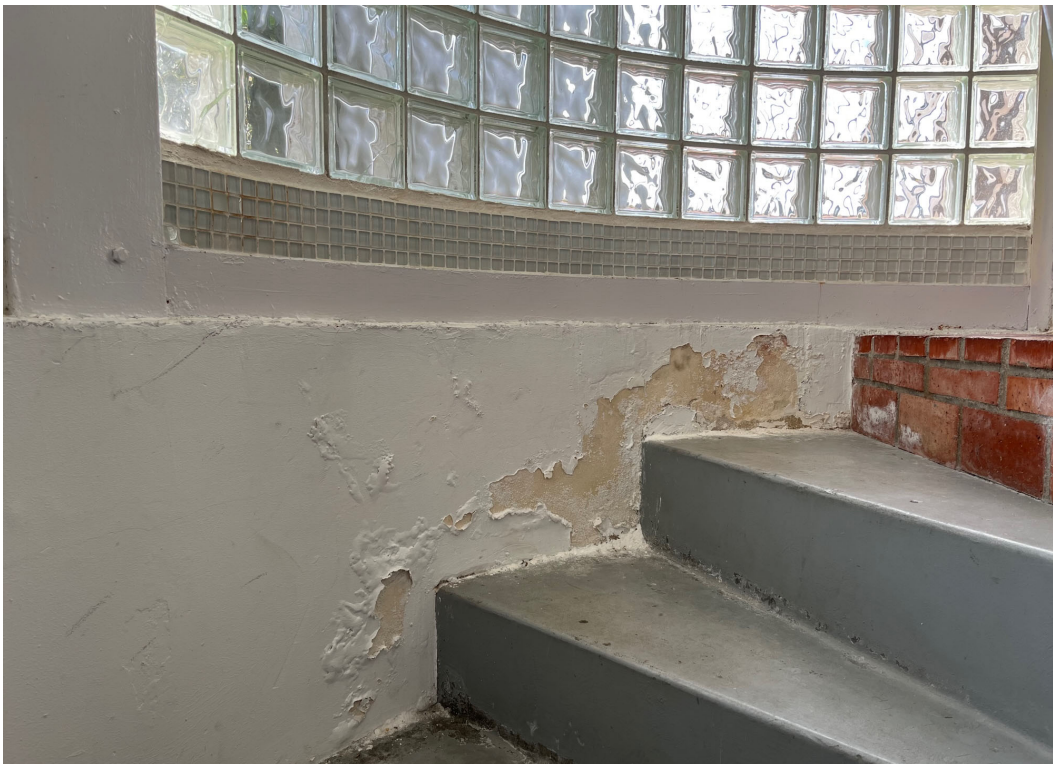
Photo 36: Wall damage at the base of the curved glass block wall in Unit 2689. Moisture is seeping through the CMU foundation wall and the bottom row of glass blocks are covered with non-historic tile on the interior to conceal damage.
