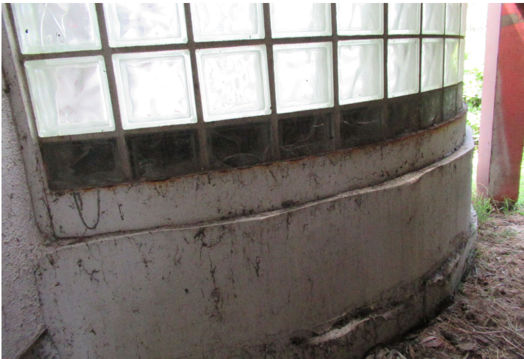
Photo 8: The base of the curved glass block wall at Unit 2689 showing the rusted steel sill and damaged/blocked bottom row of glass blocks.
