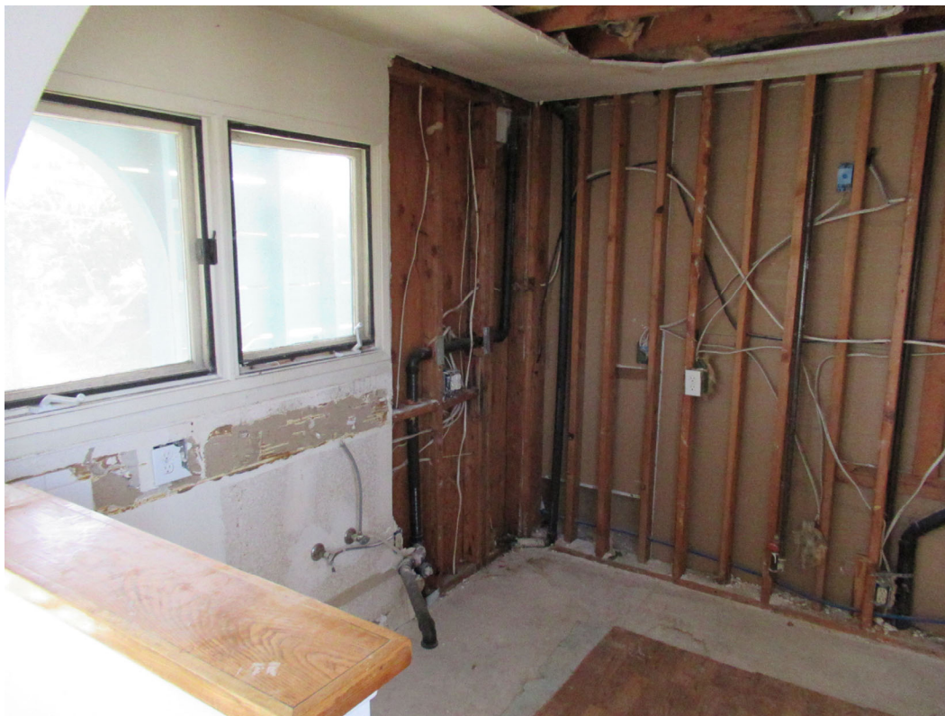
Photo 18: Missing cabinets, finishes, appliances, and fixtures Kitchen C.
