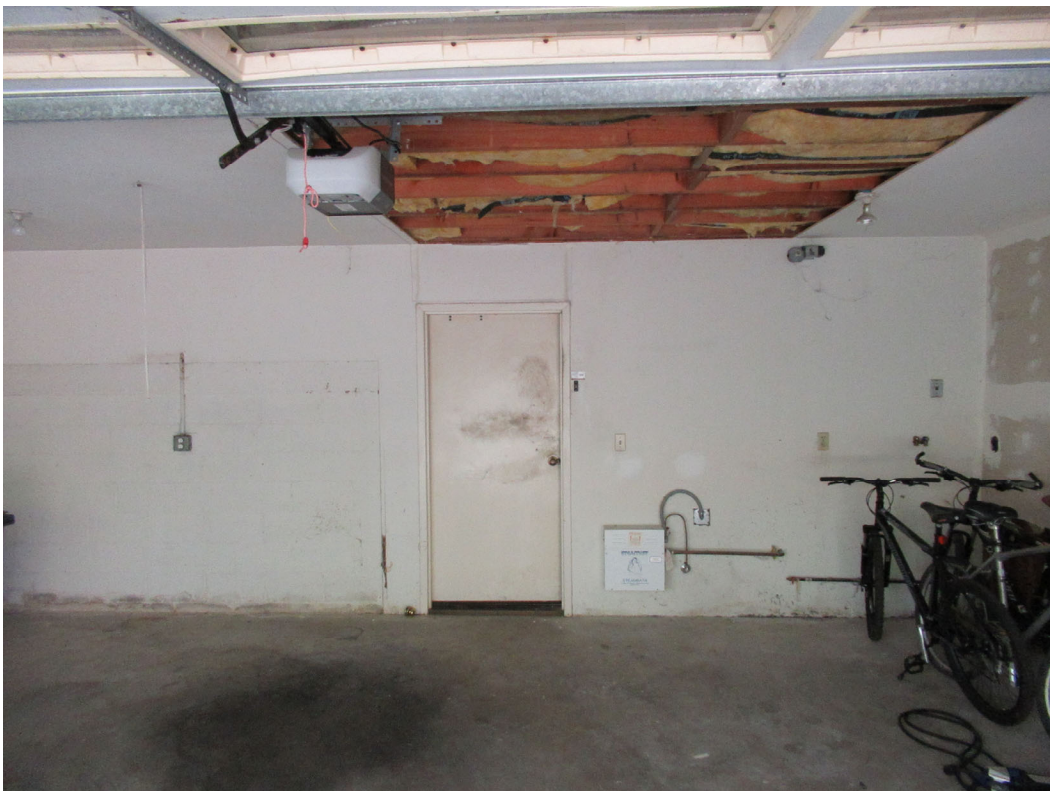
Photo 12: The garage at Unit 2685 showing missing ceiling finishes and efflorescence at the base of the east wall.
