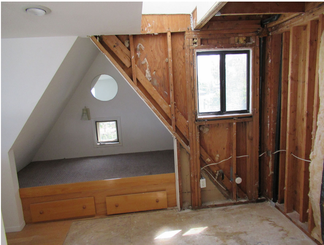
Photo 24: Damaged/missing wall and floor finishes at Mezzanine C.
