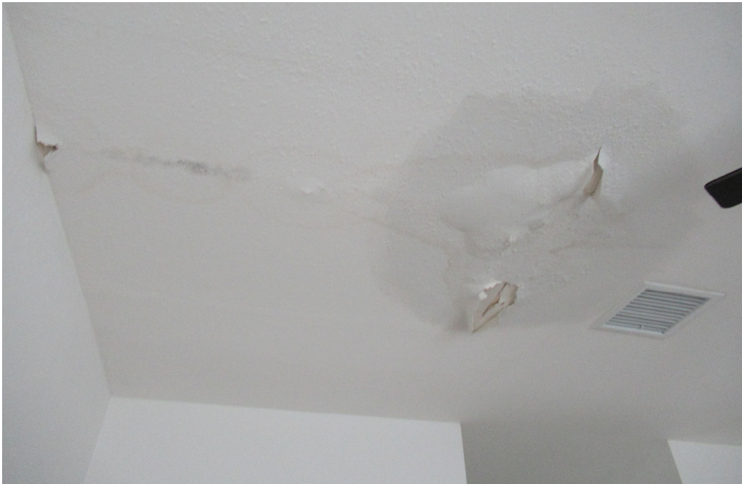
Photo 31: Water damages at the ceiling of Bedroom 2B.
