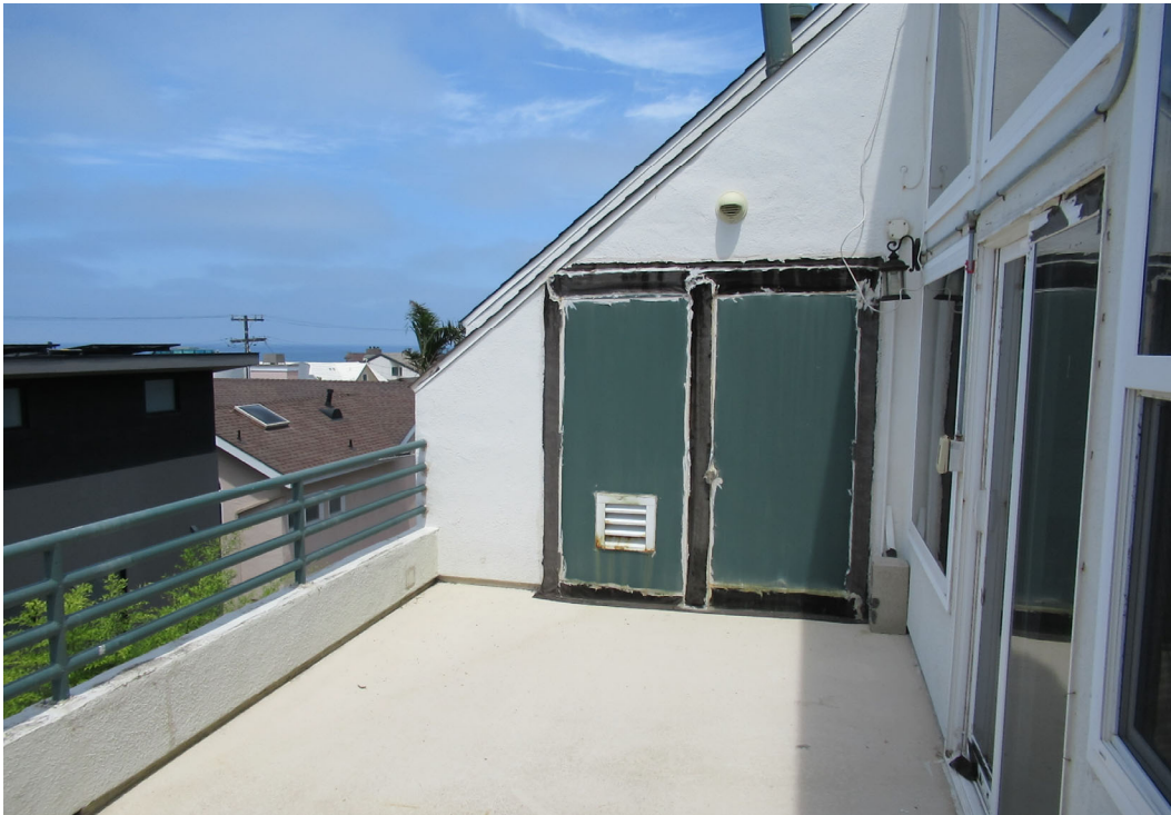
Photo 35: Balcony B showing damages/sealed double doors leading to the mechanical closet.
