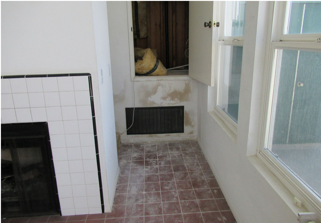
Photo 23: Damaged/stained wall under a mechanical closet on the south wall of Living Room C.
