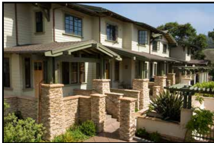
Change in color and texture along wall surface
