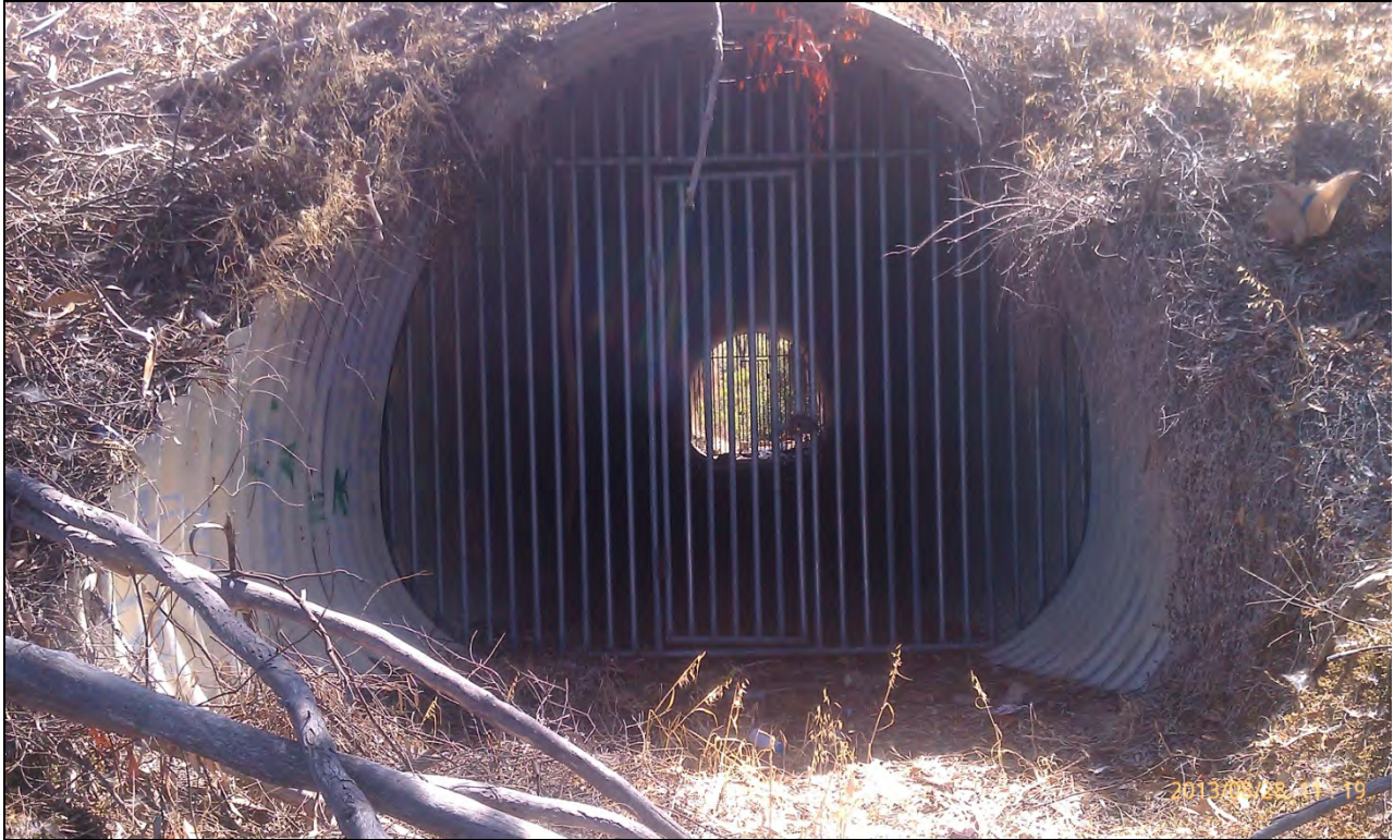
M1-2 – west side facing east, showing locked gate at both ends, August 2013.
