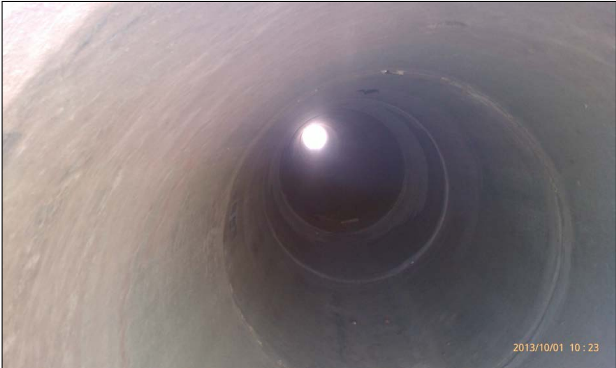
CC3-3b, north side entrance facing toward undercrossing showing long, narrow pipe, Oct 2013.
