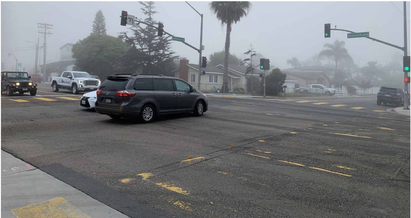
Faded crosswalks at this wide intersection at Jefferson Street/Tamarack Avenue
