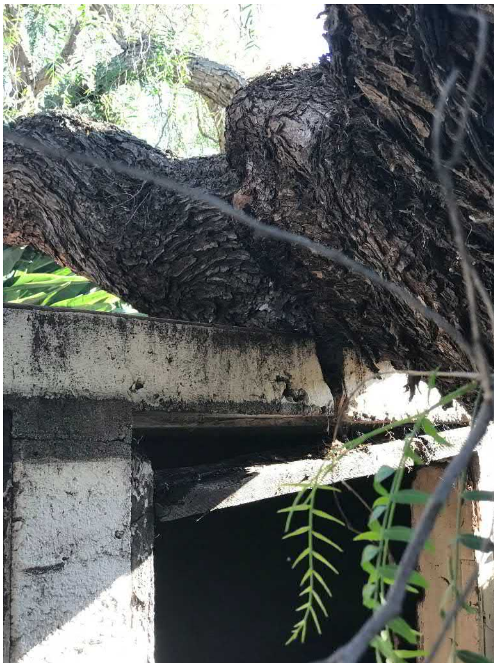
Broken door frame and crack in the concrete roof. 2018
