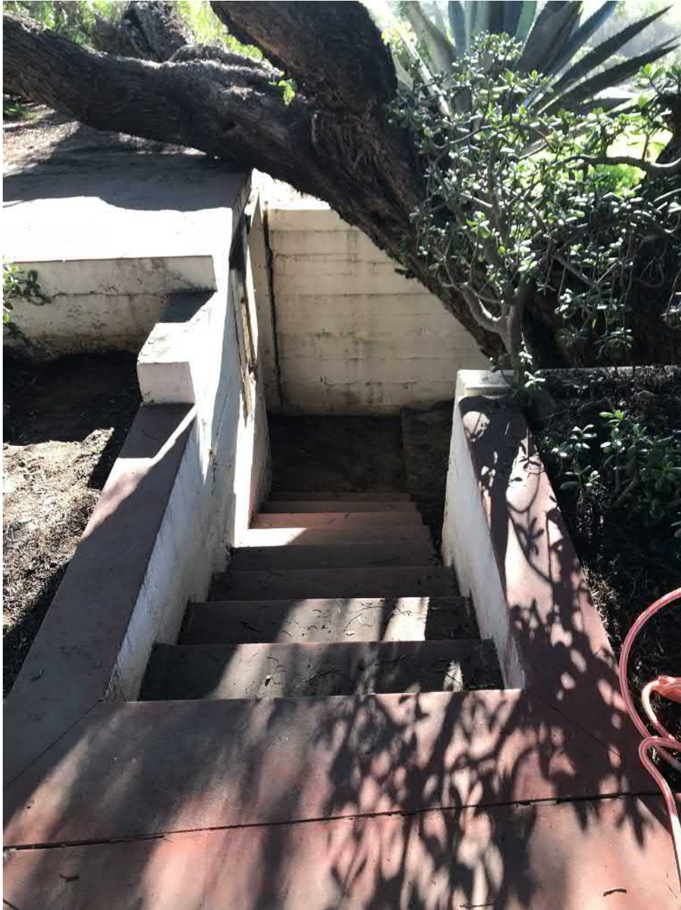
A 16" branch resting on the storeroom. The crack is between the two branches. 2018.
