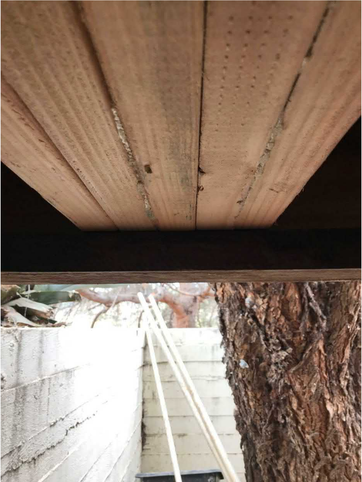
Laminated beam supporting the roof and resting on the new door frame. 2018
