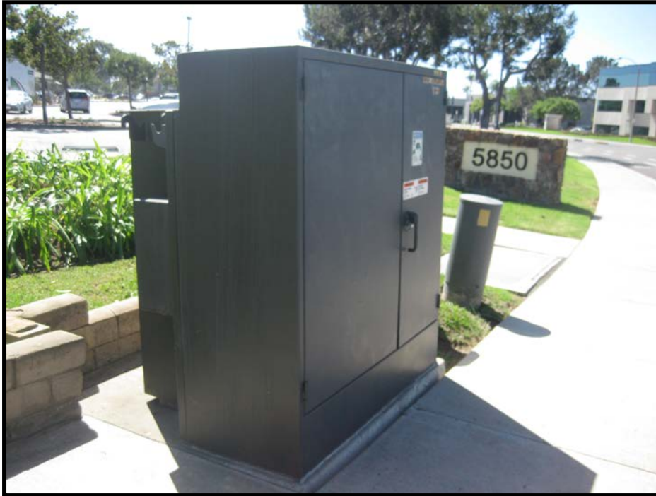
View of the pad mounted transformer adjacent to the northwestern property boundary.
