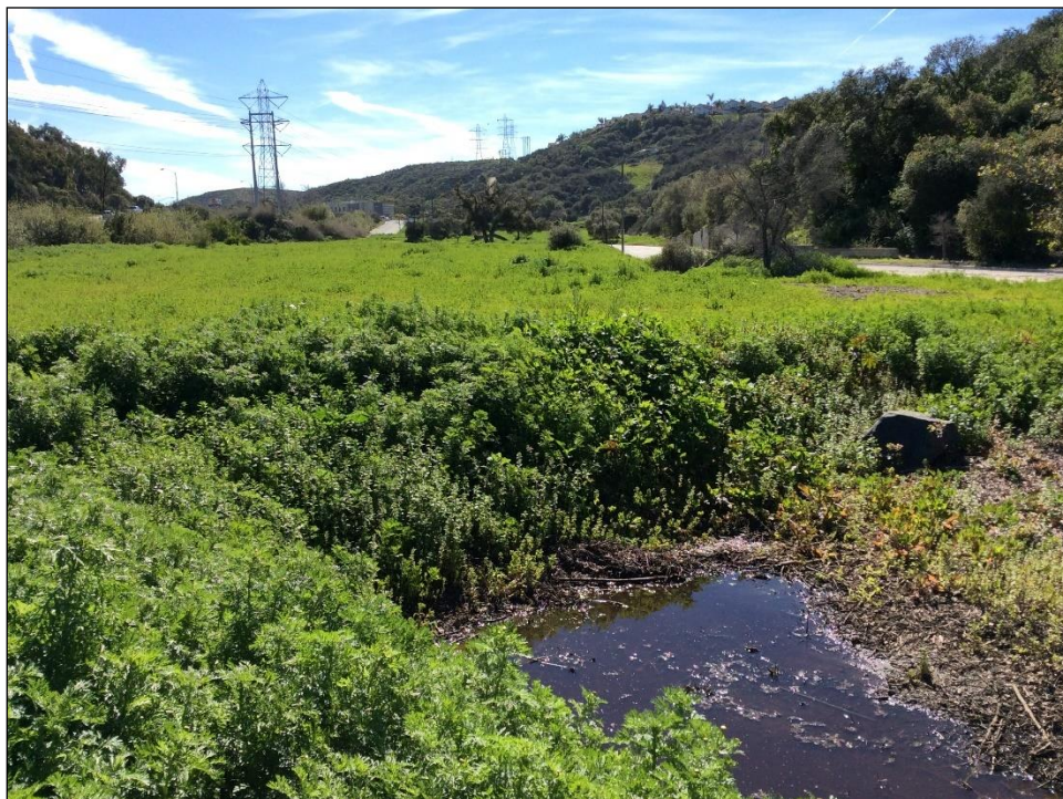
Figure 6 Depression in northern portion exposing fill material, view facing southeast.
