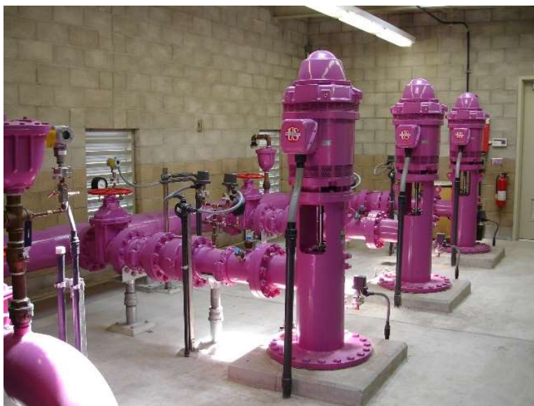
Calavera Hills Pump Station (60 HP)
