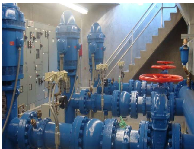
The 125 HP Bressi Potable Water Pump Station
