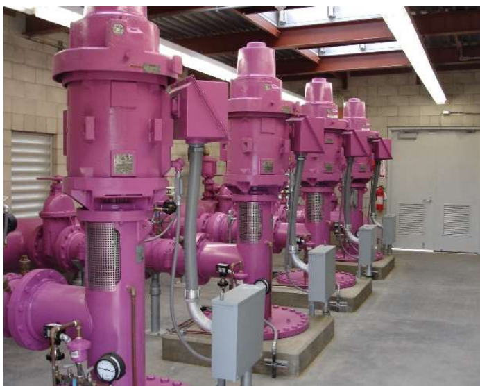
The 150 HP Twin "D" Pump Station, which helps deliver recycled water to CMWD customers.
