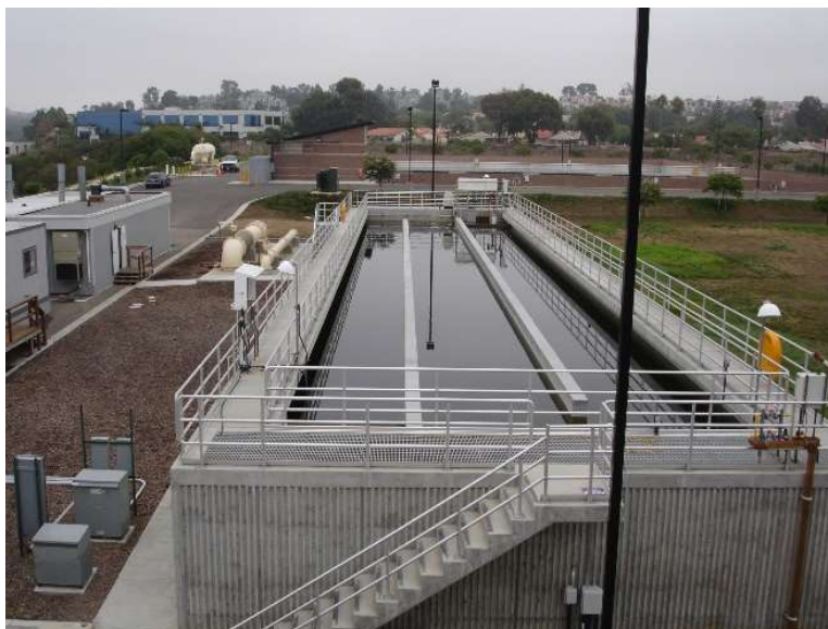
Chlorine contact basin at the existing Carlsbad WRF
