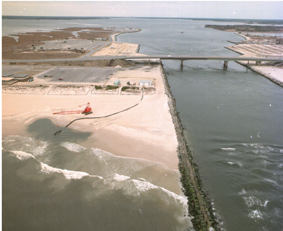
Figure 2-21. Indian River Inlet Sand Bypass System (USACE, 2020)
